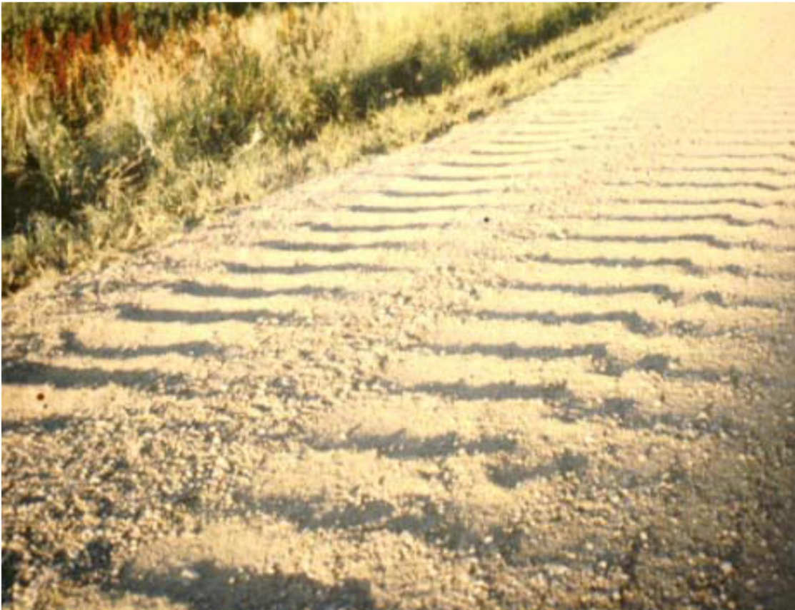
Figure 1: Corrugation or Washboarding
